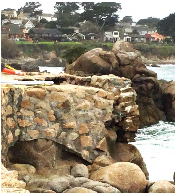
A five-foot piece of retaining wall broke away at the foot of Naiad Street (off Mermaid) in a recent storm. Even the yellow caution tape has since blown down. Photo by Beth Penney.
