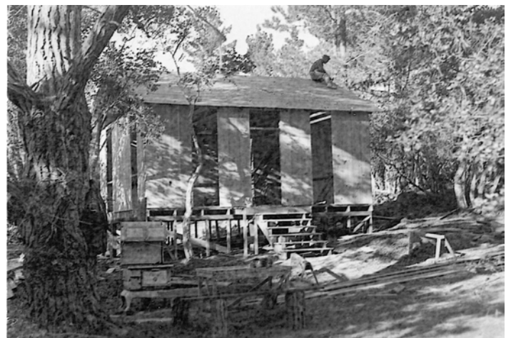
The Fox home under construction in 1940. Note the stove at lower left.
